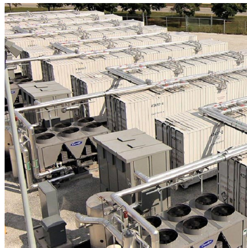
AES Battery Storage | AES
